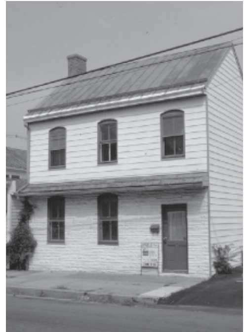
Frequently, the installation of artificial siding results in the removal of historic elements like brackets and porches.
