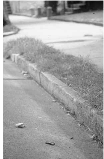
Limestone curbs are a unique and valuable feature to the streets of the historic district.
