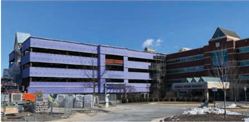
Winchester Medical Center built an addition to the Medical Office Building, totaling 42,000 square feet. The project was approved administratively.
